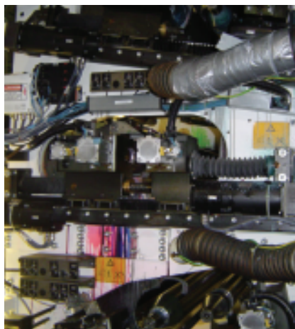
DECK leaking on mandrel below
