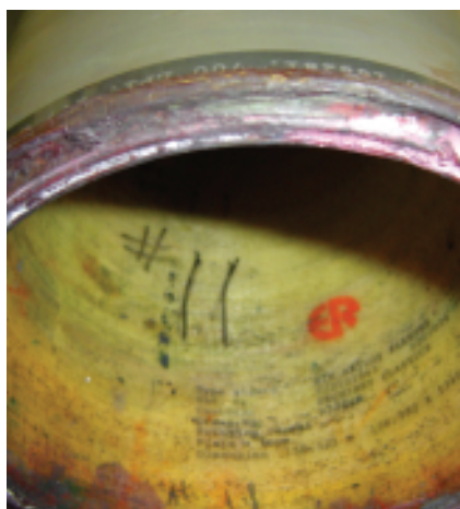
END wear with delamination of layers
