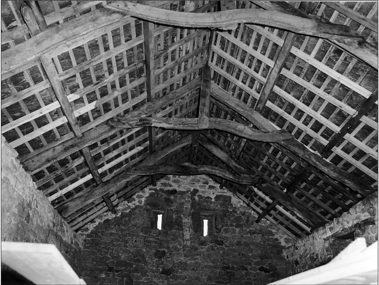
The roof of the shippon, reconstructed in the 18 th of early 19 th century, when the wall-heads were built up to allow the shallower pitch necessary for slate; after repairs of 1977-78.
