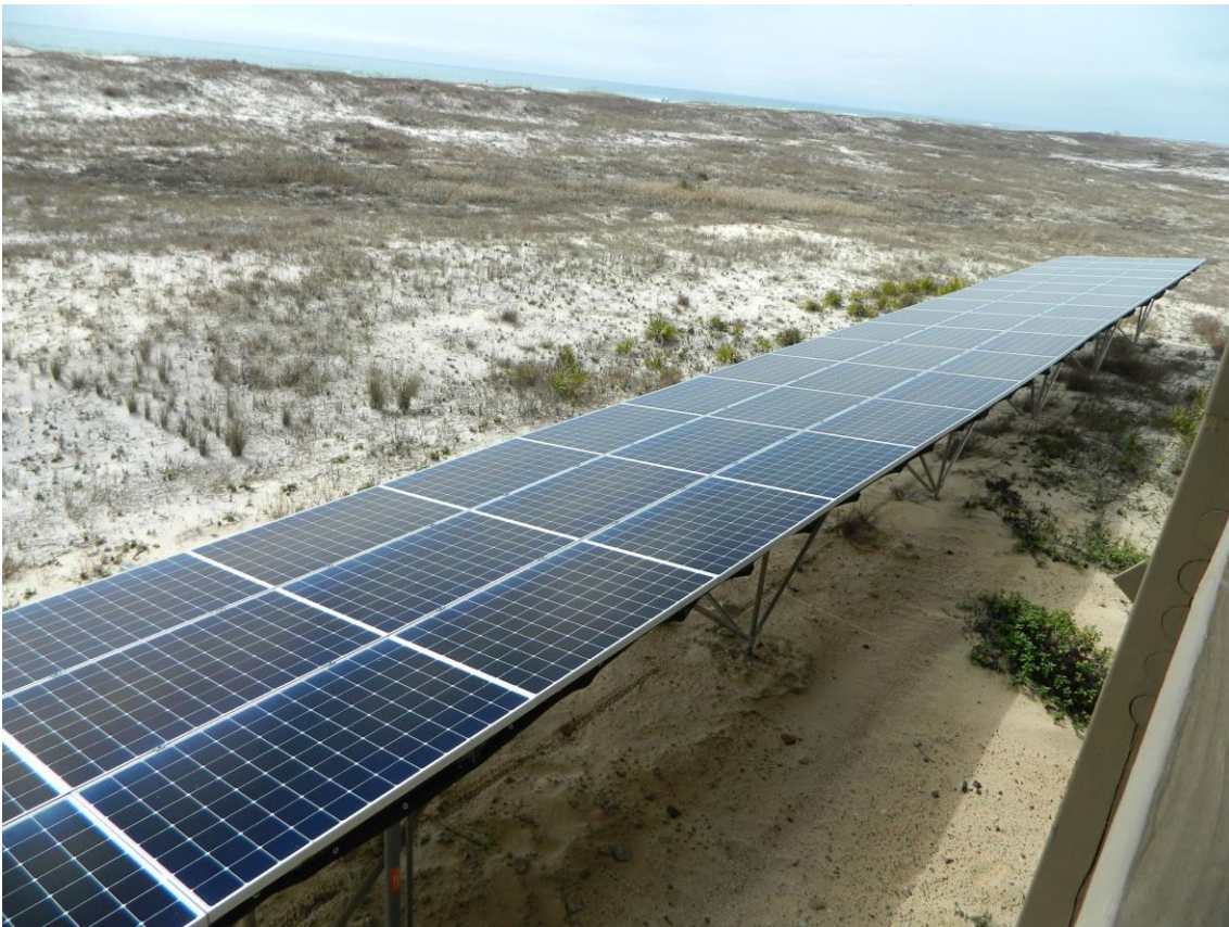
Figure 18. Solar panels are used to power the Interpretive Center (LeBleu, 2022).
