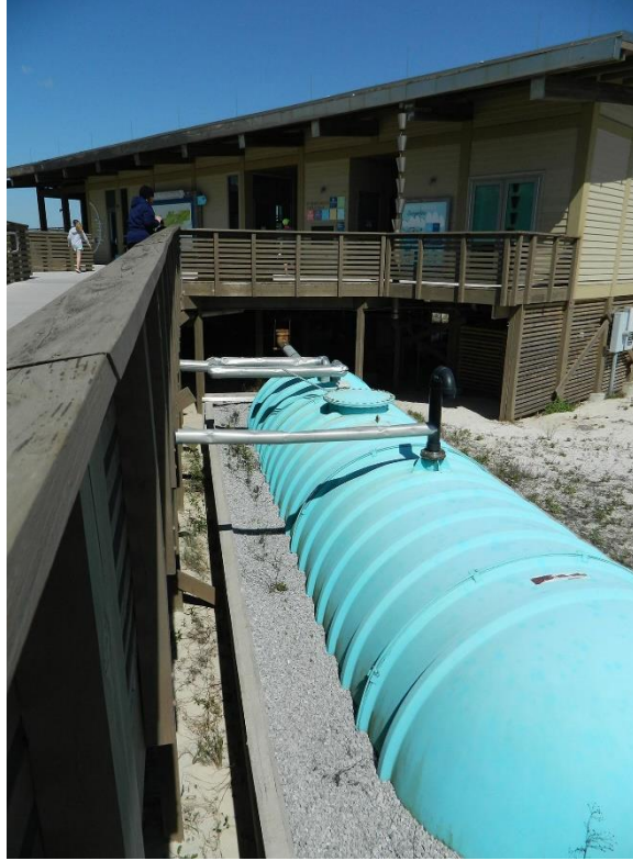
Figure 4. 11,000-gallon (41,640 L) cistern at the GSP Interpretive Center (LeBleu, 2022).
