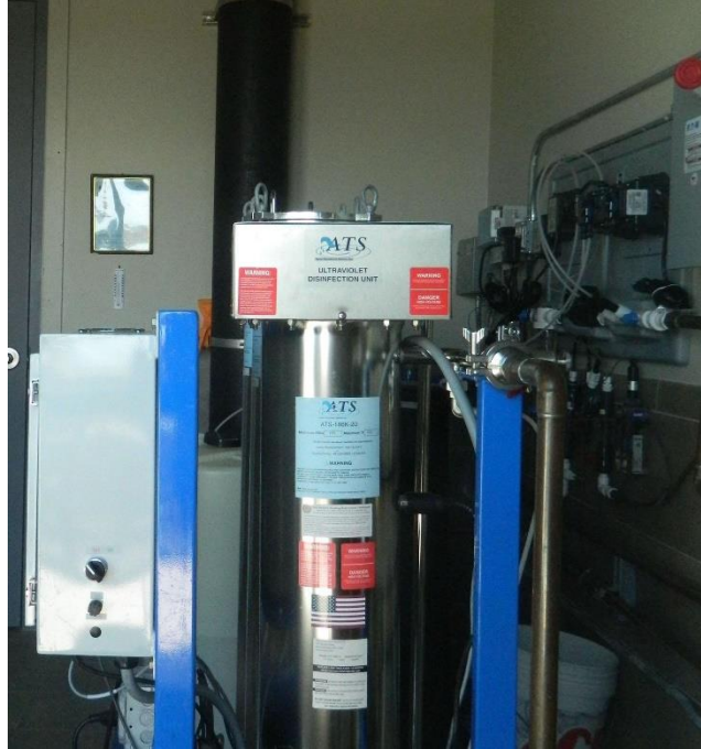
Figure 6. Ultraviolet water disinfection system (LeBleu, 2022).
