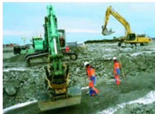
Construction work for the Ormen Lange field, Norway Ormen Lange is Europe's second largest offshore gas field. It is situated in an area where climatic and oceanographic conditions make it one of the most challenging developments in the world.
