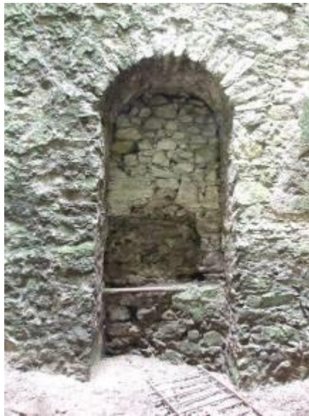
Blocked entrance door to tower
