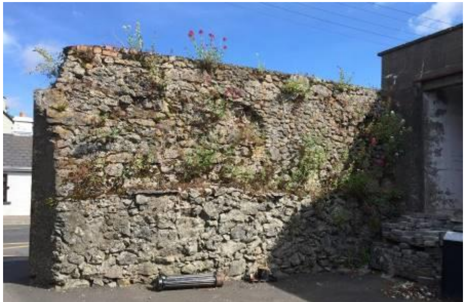
Inner face of wall showing vertical section formerly hidden under earthen bank
