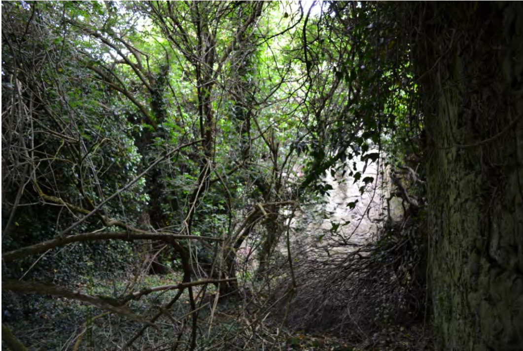
Plate 11: Severe vegetation growth over an extended period threatens the integrity of upstanding remains - as at this church in Clonkeen (L039). It would now be a large task to attempt to restore the burial ground to a state where it could be accessed and regularly maintained.
