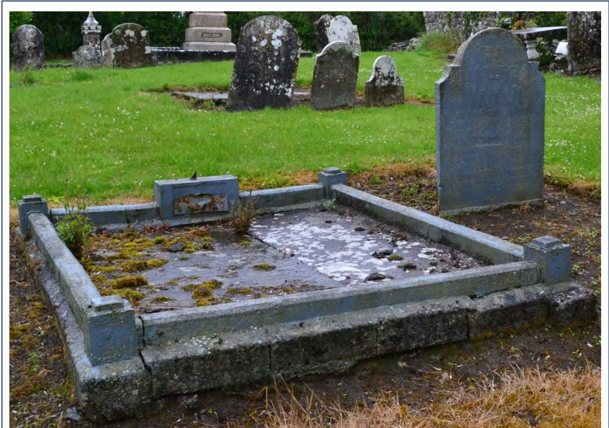
Plate 10: The temporary coat of blue-grey paint over the otherwise well-preserved 250 year old headstone is out of character with its own origins as well as the other memorials in the burial ground.
