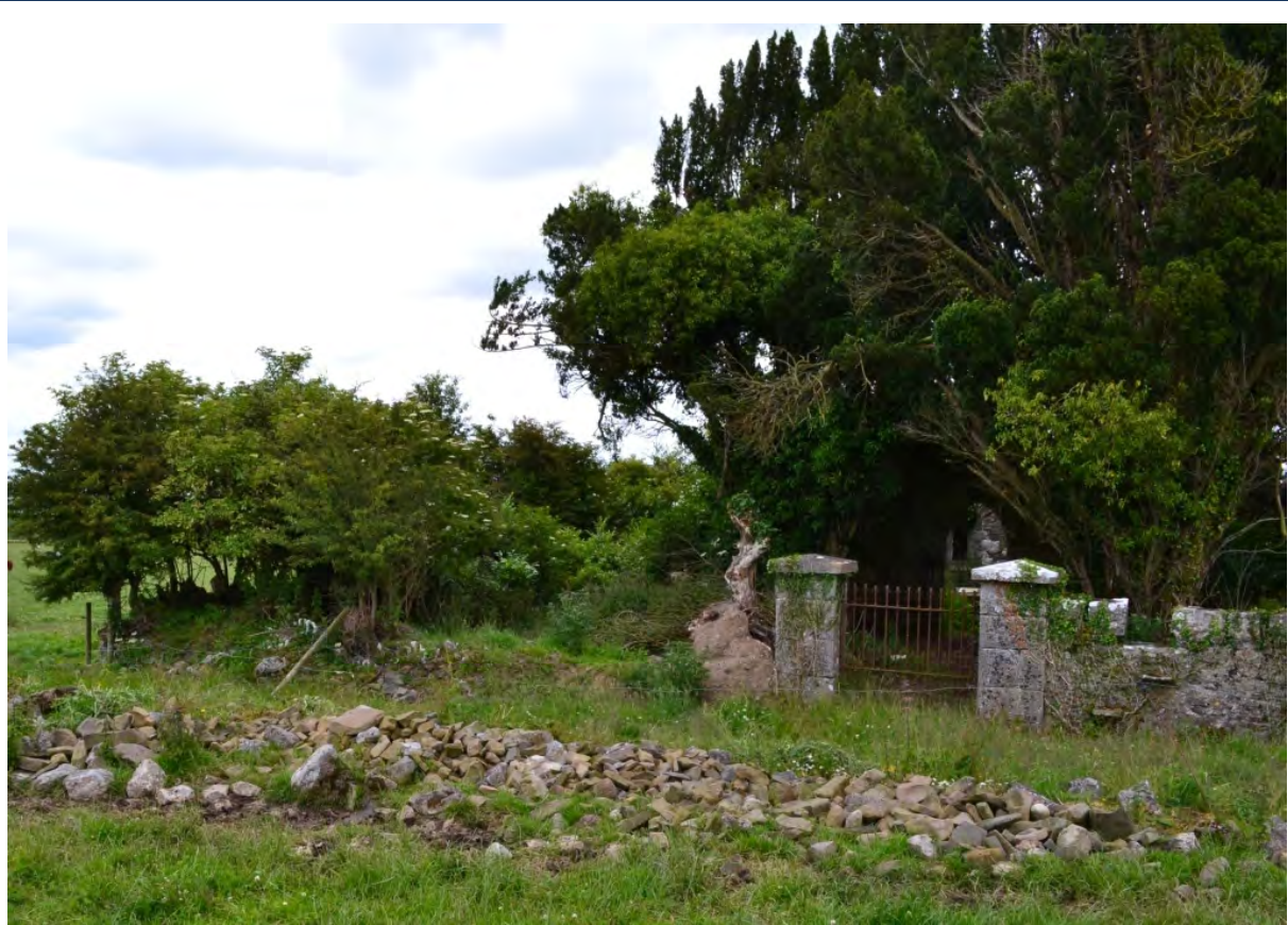
Plate 13: Repairing this section of enclosure wall at Cremorgan (L047) would greatly benefit the long term conservation of the burial ground in addition to keeping cattle from the poisonous yew trees that occupy a traditional place in the landscape.
