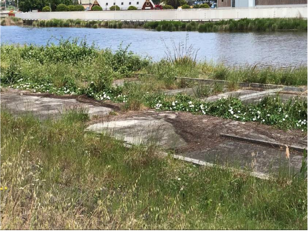
Plate 2 View from southern bank of North Esk River overlooking old rowing club house foundations.
