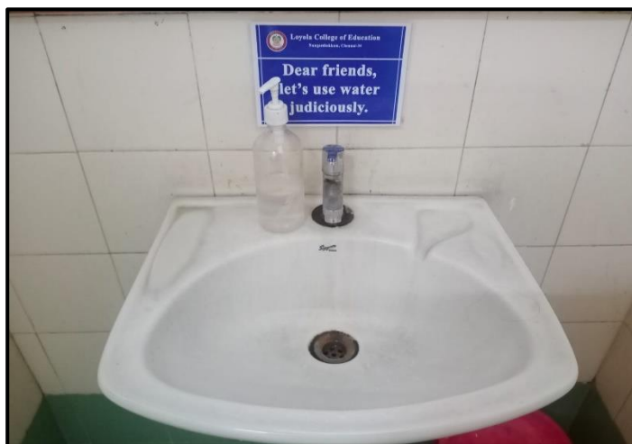
Proper Maintenance of Taps without any leakages in LCE Campus, Chennai , TN
