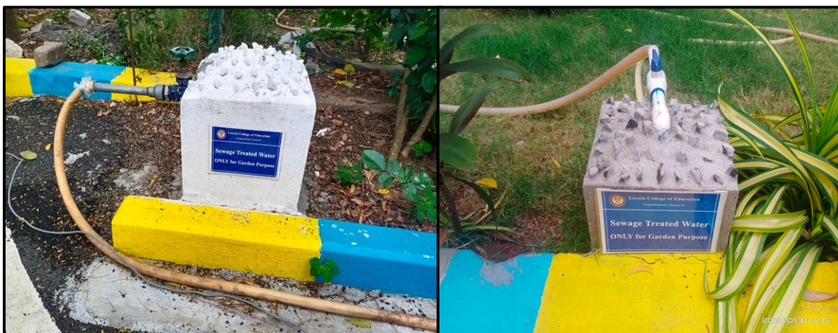
STP Observed at LCE Campus, Chennai, TN
