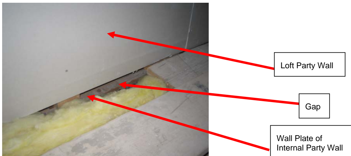
Figure 8 – Gap between Top of Internal Party Wall and Party Wall in Loft
