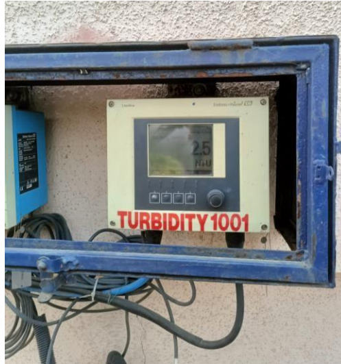
Figure 13: Quality of water is monitored and controlled by control systems
