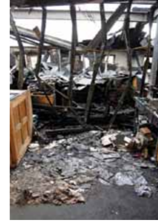
Difrod y tân / Fire damage
