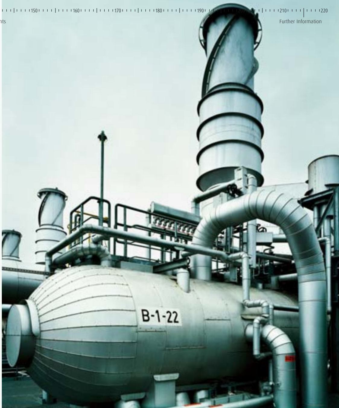
An essential part of an olefin plant: the residual heat in the high pressure steam boiler is used to drive the turbines.
