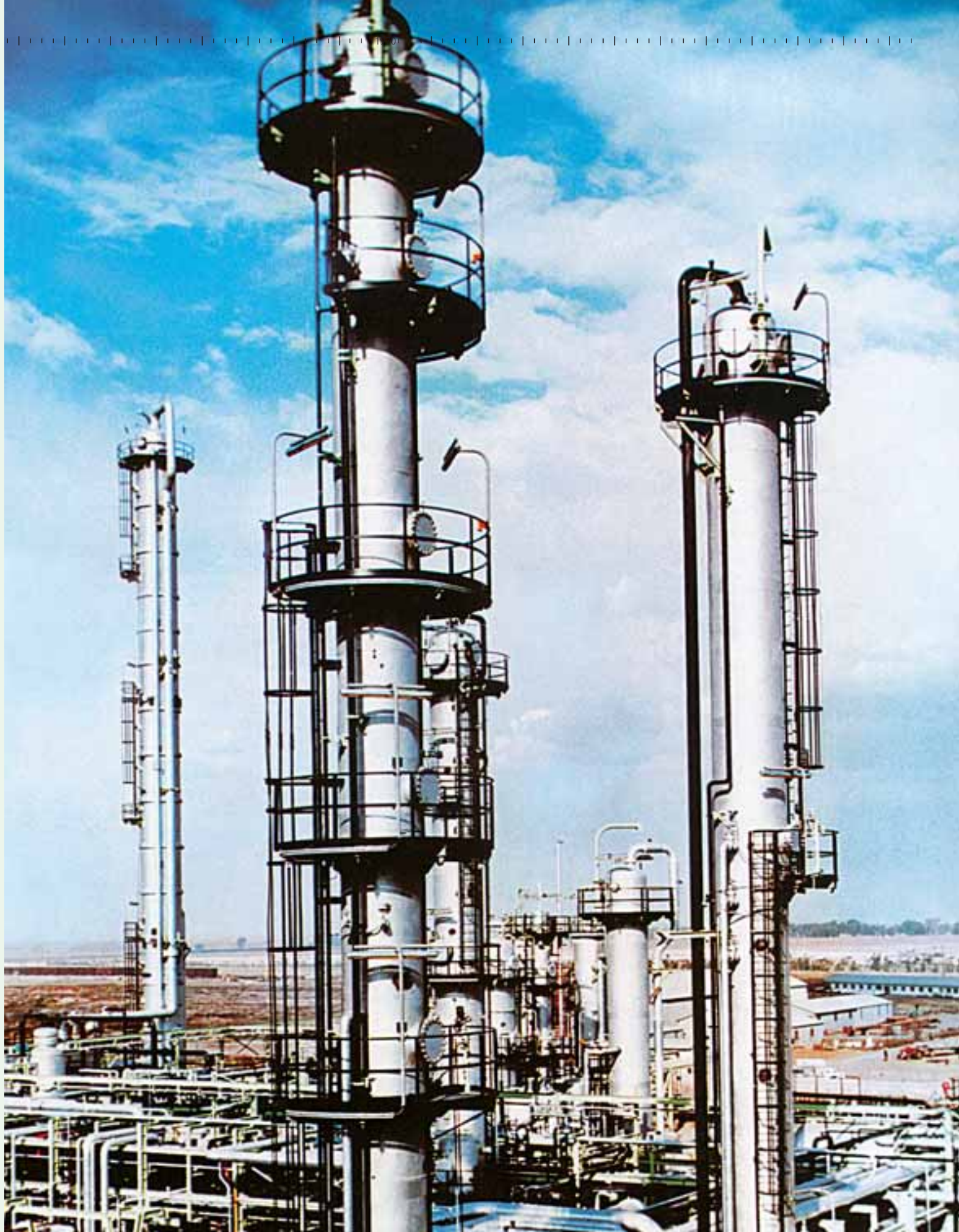
Partial view of a petrochemical plant constructed by Linde in South Africa.
