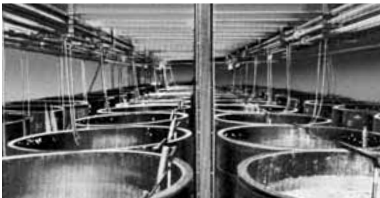
Fermentation cellar of a brewery with natural convection cooling.
