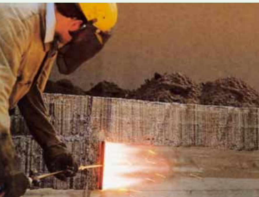
Gas application in the construction industry: Flame descaling with autogenous flame for finishing concrete surfaces.
