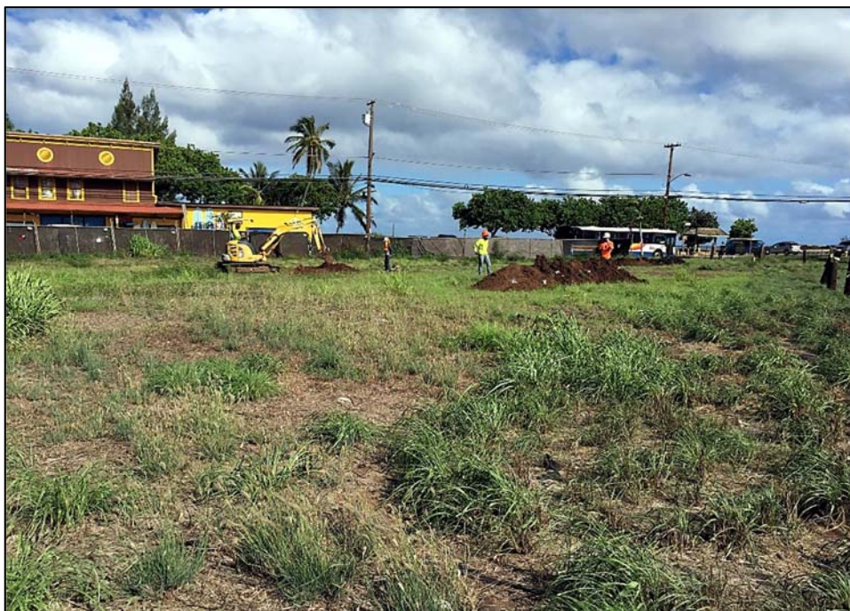
Figure 16. Overview of the parcel, showing light vegetation. Orientation is to the northwest.
