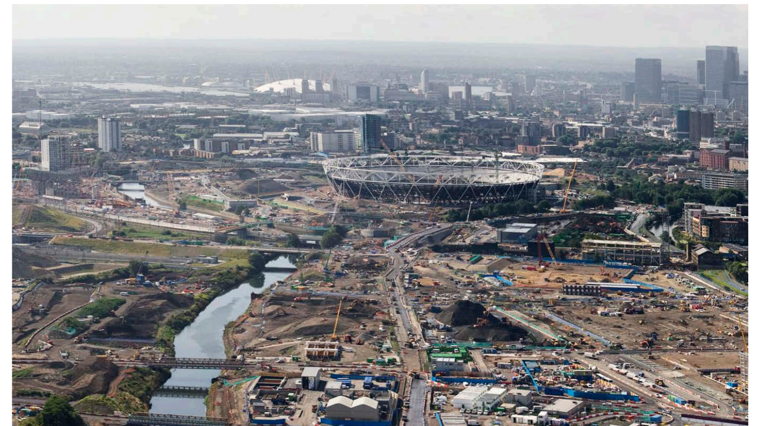
London 2012 Olympic Games. Overall the sustainable approach adopted for land rehabilitation resulted in: 246 hectares of land rehabilitated; 98% of demolition material recycled; 2.2 million m 3 soil excavated and 80% of soil re-used. Source: Atkins and the London 2012 Games
