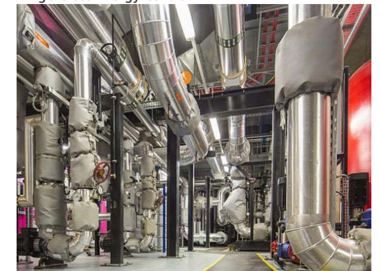
King's Cross Energy Centre
