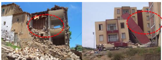
Figure 7: Collapse by type of structure, on the left a masonry building and on the right a collective building with reinforced concrete at Dellys (source: Akreche design office, 2003)
