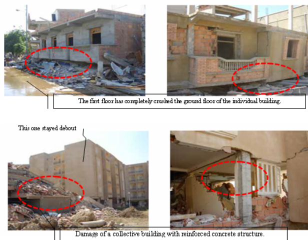
Figure 11: We observe two cases, the total disappearance of the ground floor of a private residential building with 1 to 2 floors, in the second case total disappearance of a collective building with 3 to 4 floors (Source: Japan Association of Earthquake Engineering (JAEE) et al., 2004).
