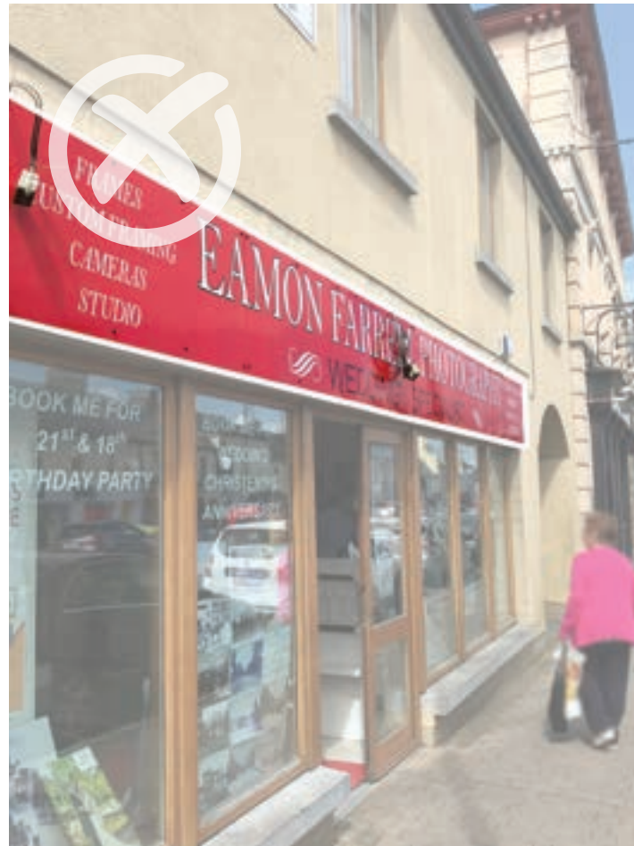
Fig. 13. Shallow shopfront fascia with unnecessary additional text.
