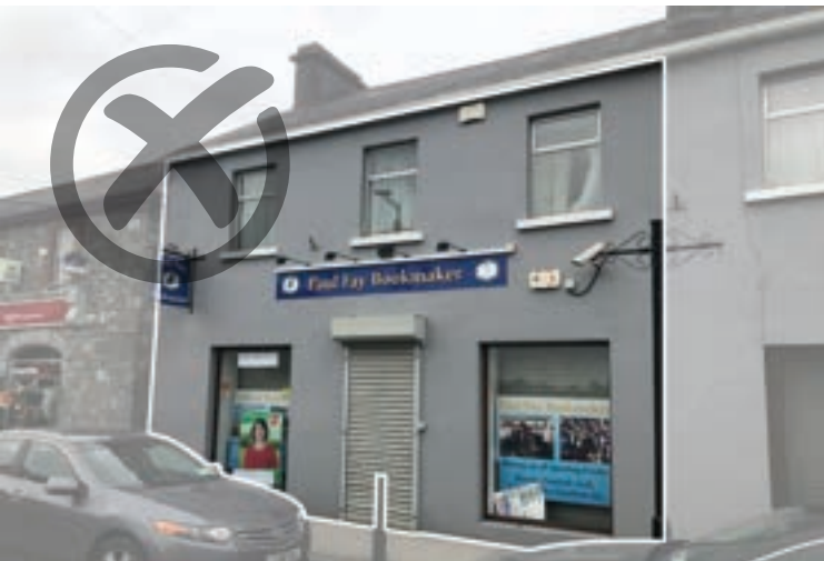
Fig. 22. Bland and uninteresting bookmaker shopfront with unsuitable, externally mounted security shutter and shutter box.
