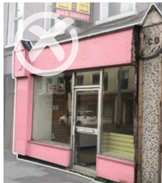
Fig. 20. Lurid colour timber shopfront over decorate original.
