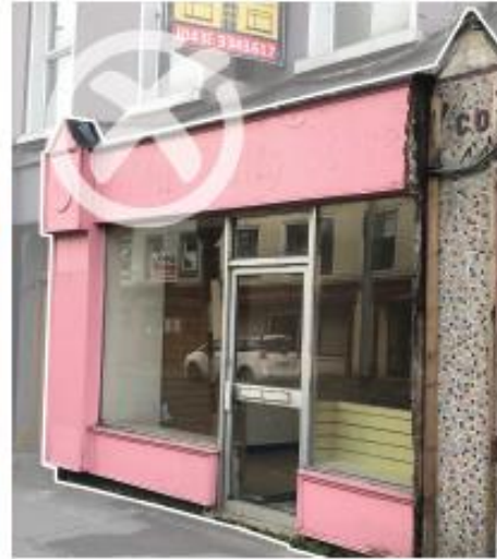
Fig. 20. Lurid colour timber shopfront over decorate original.
