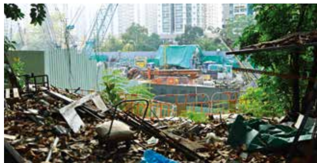
該住宅項目距離龍窯僅 30 米，於 2020 年開始地基工程。 The housing project, just 30 metres from the kiln, started foundation works in 2020.
