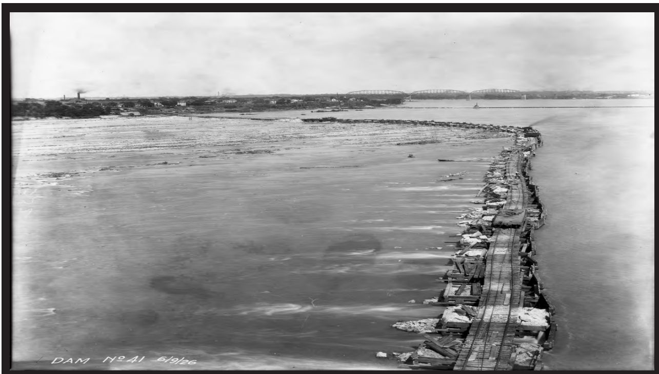
The nearly completed box cofferdam dries the Falls for dam construction. In the background is Jeffersonville. (Corps of Engineers)
