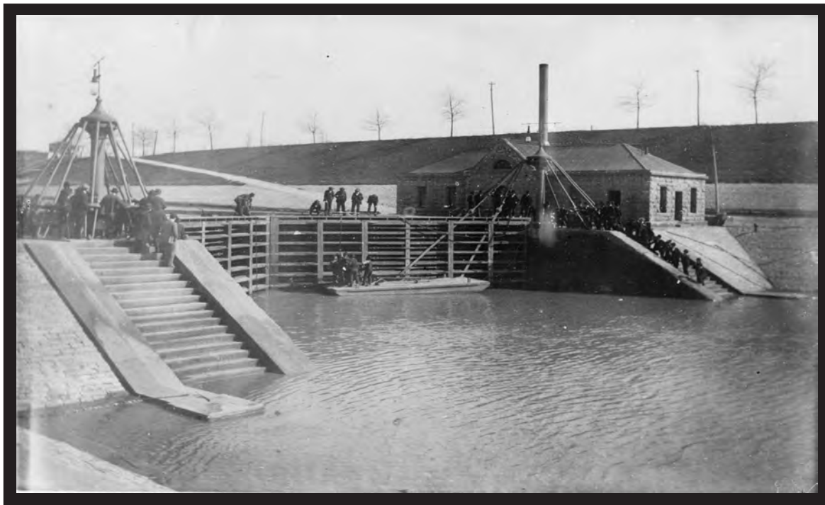
Repairs underway at the Scowden lockgates in 1884. Note the kingposts used to suspend the lockgates. (National Archives)
