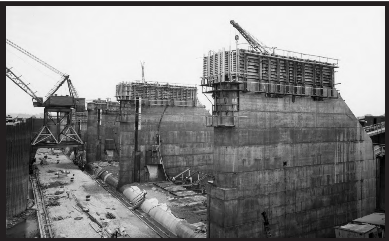
Concrete placement in the Tainter gate piers shown in this May 1961 view. (Corps of Engineers)
