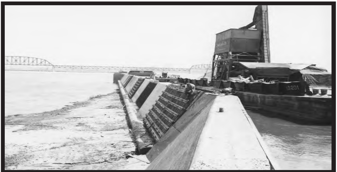
With forms in place, concrete placed in the Boule sections converted the movable to a fixed dam. (Corps of Engineers)
