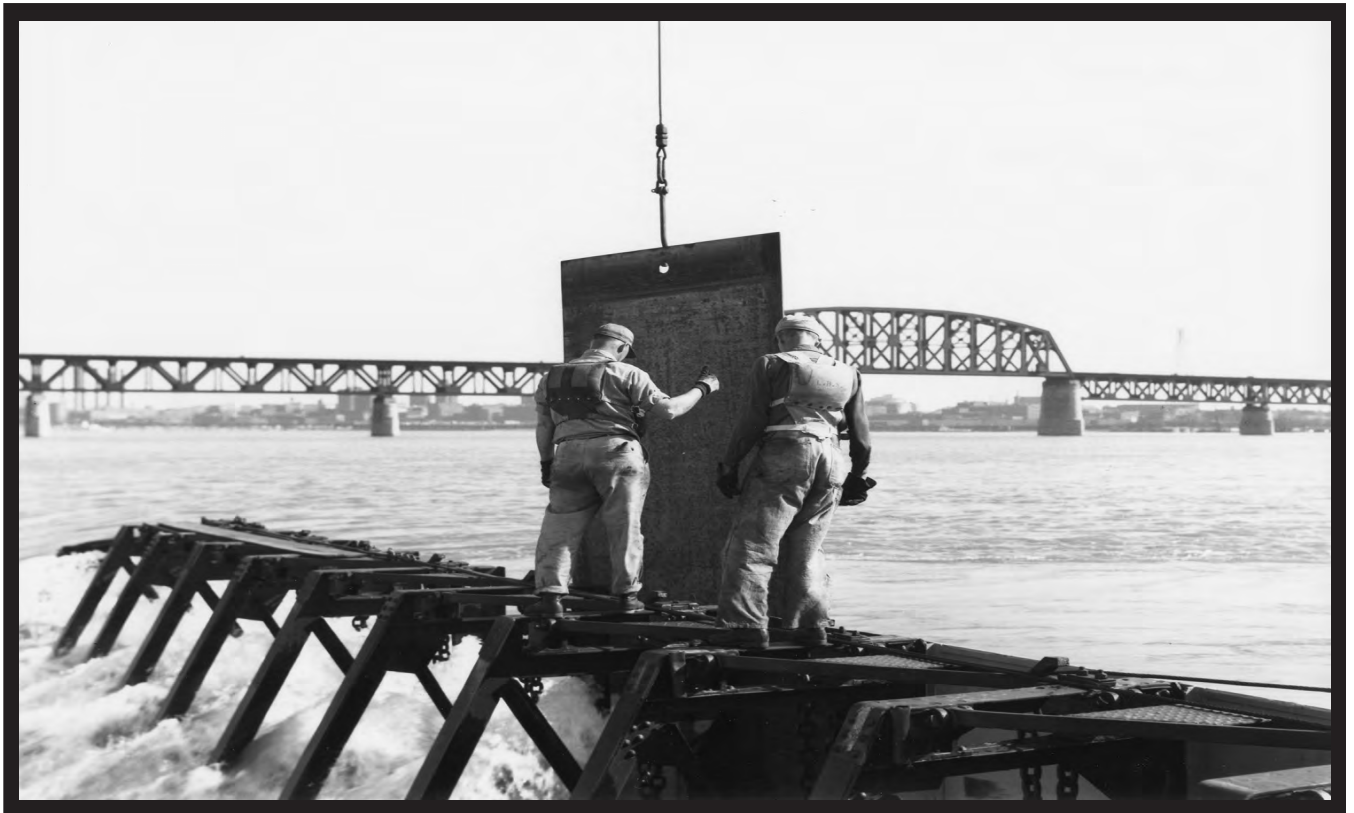
Workers guide the metal shutter down the front of the Boule trestles. This was hazardous duty and at least four District personnel lost their lives in this service. (Corps of Engineers)
