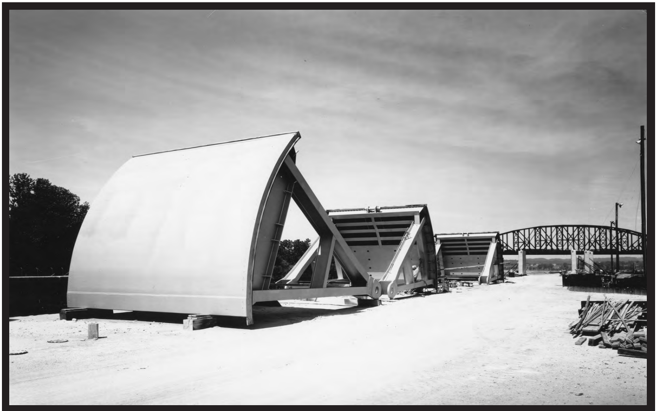
Tainter gates assembled and ready for installation in the 1200-foot lock's filling and emptying culverts. (Corps of Engineers)
