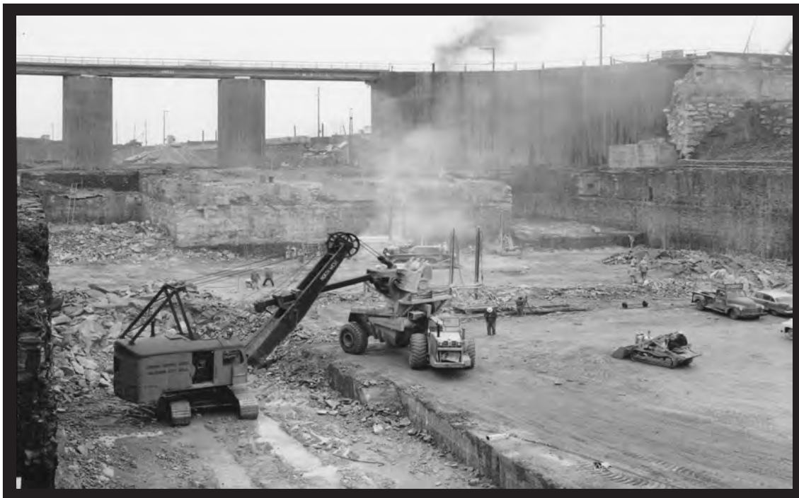
Rock excavation to open space for the McAlpine Lock. The temporary bridge in the background carried vehicles to Shippingport island during construction. (Corps of Engineers)
