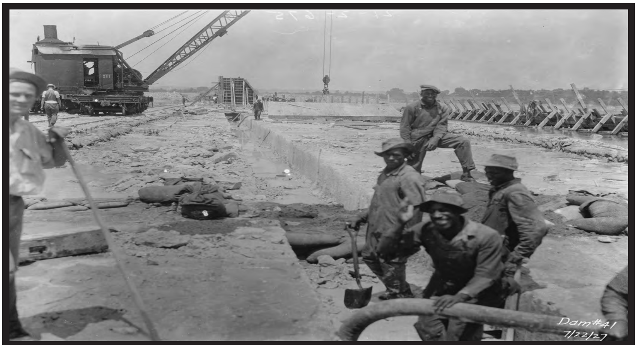
Workmen excavating a key trench into the Falls rock as foundation for the new dam. (Corps of Engineers)
