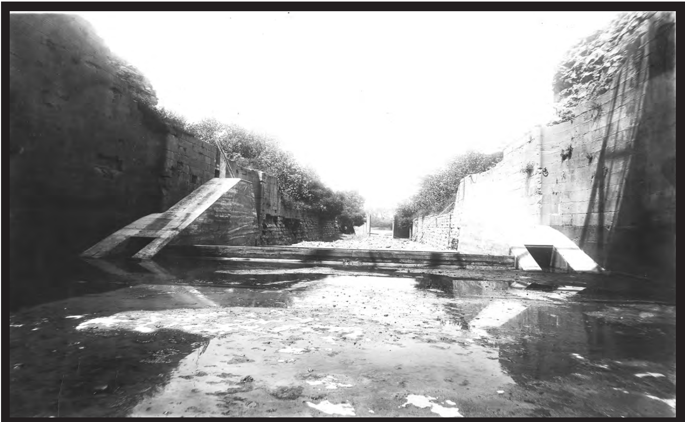
The original lock chambers often filled with mud and debris, forcing closure for its removal. (Corps of Engineers)
