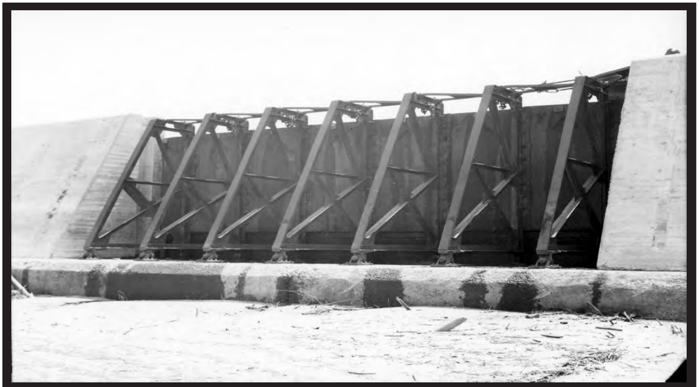
A 1952 view of the Boule dam section with shutters installed before forms were placed to hold concrete. (Corps of Engineers)
