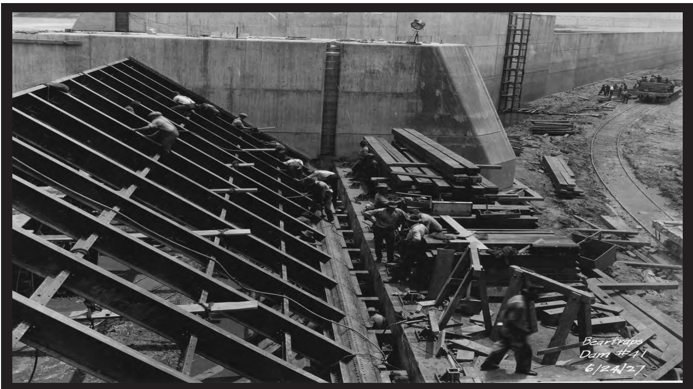
Construction of the beartraps to control minor river flows. (U.S Army Corps of Engineers)
