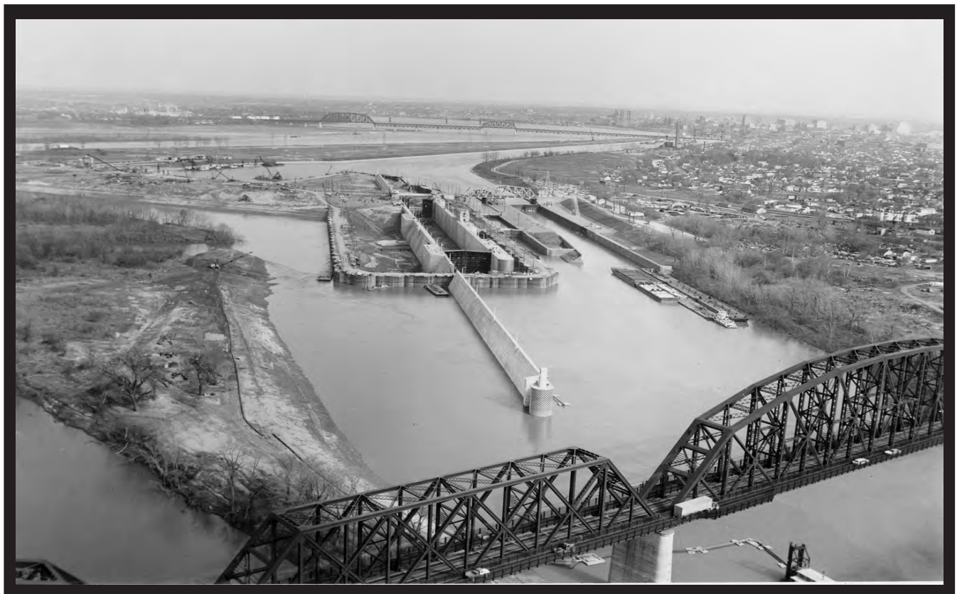
Looking upstream at the cellular steel cofferdam around the new 1200-foot McAlpine Lock while the Scowden Locks and Lock 41 continue in service. Kentucky and Indiana bridge in the foreground and Sand Island on the left. (Corps of Engineers)
