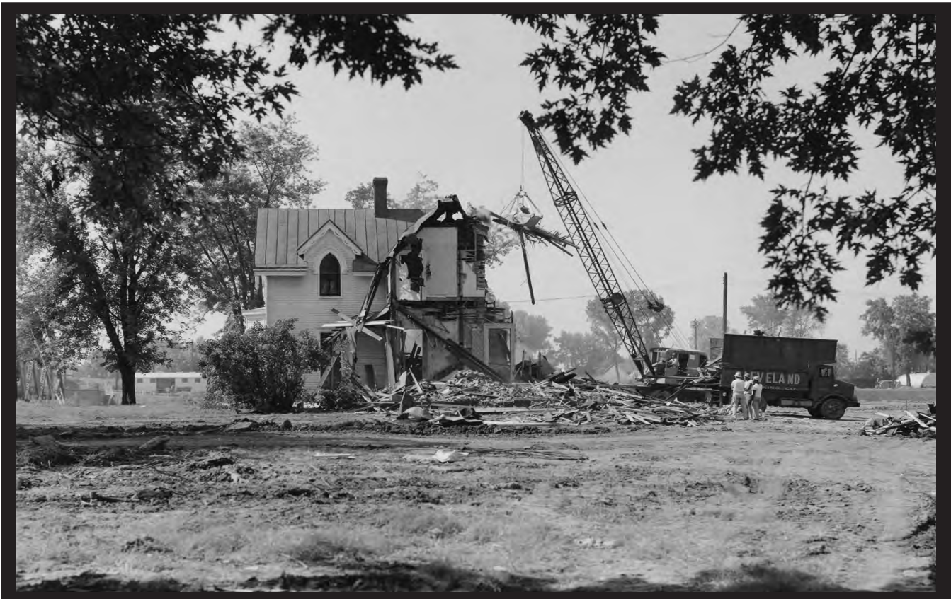
The lockmaster's house was demolished in 1958 to make way for the 1200-foot McAlpine Lock. (Corps of Engineers)
