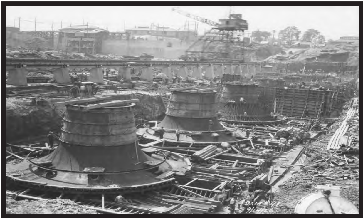
Construction of the powerhouse foundation and hydrocones in late 1926. (Corps of Engineers)
