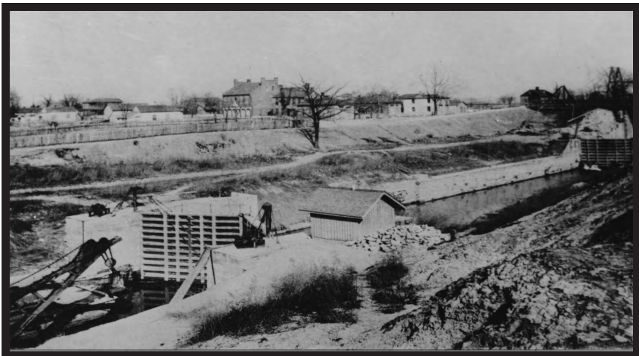
This view of the original locks of 1830 show a thriving Shippingport in the background. Note the kingposts suspending the lockgates and the dredge in the lower lock chamber at the left. (National Archives)
