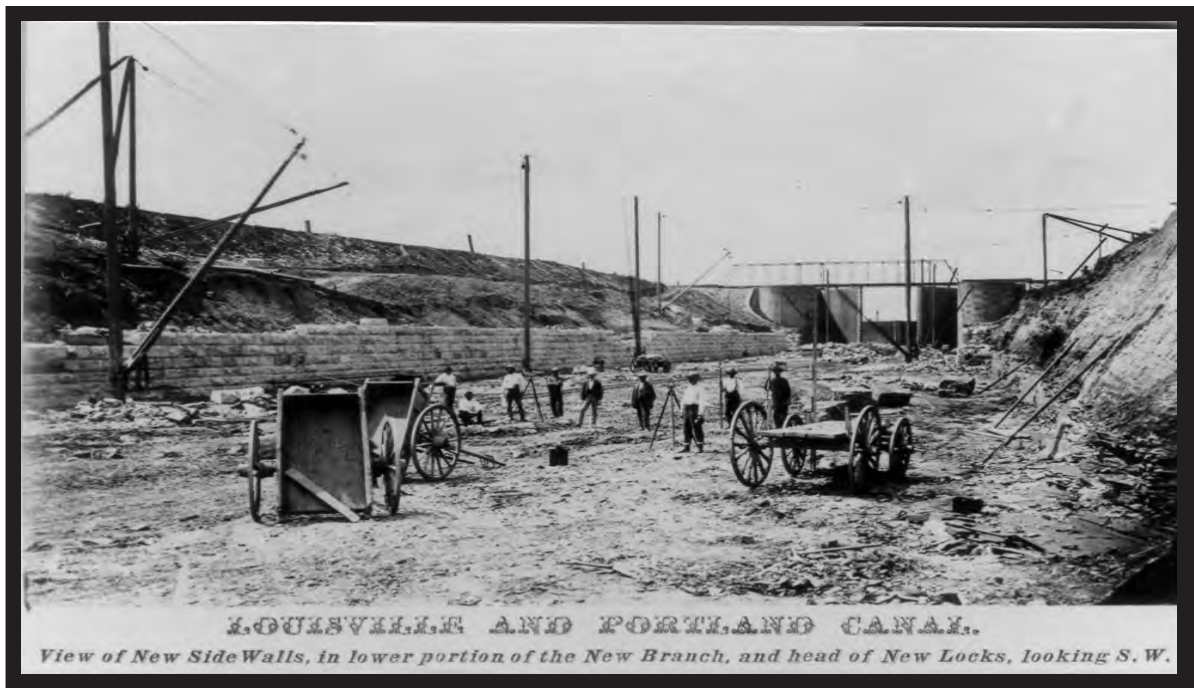
The original canal of the 1820s was built by manual labor and teams of oxen and horses. Stiffleg derricks made of timber poles and cable hoisted and moved stones into place. (Klauber Collection, University of Louisville Photographic Archives)
