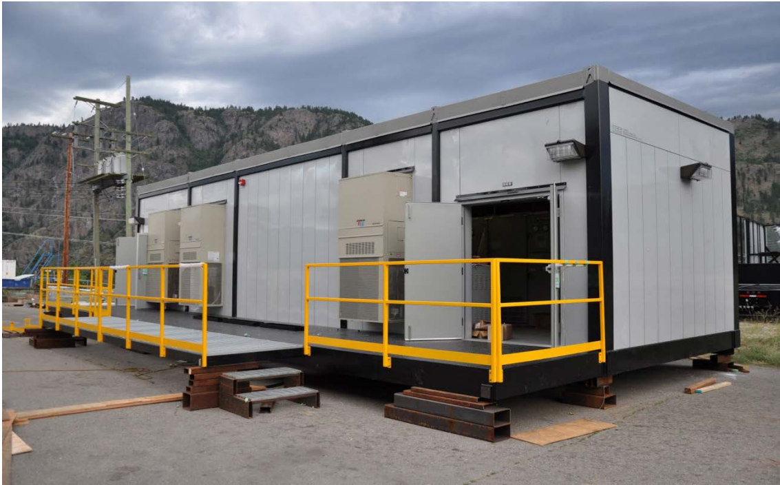
Figure 4: Photograph of MV Export switchgear and storage facility (source: Infratec).
