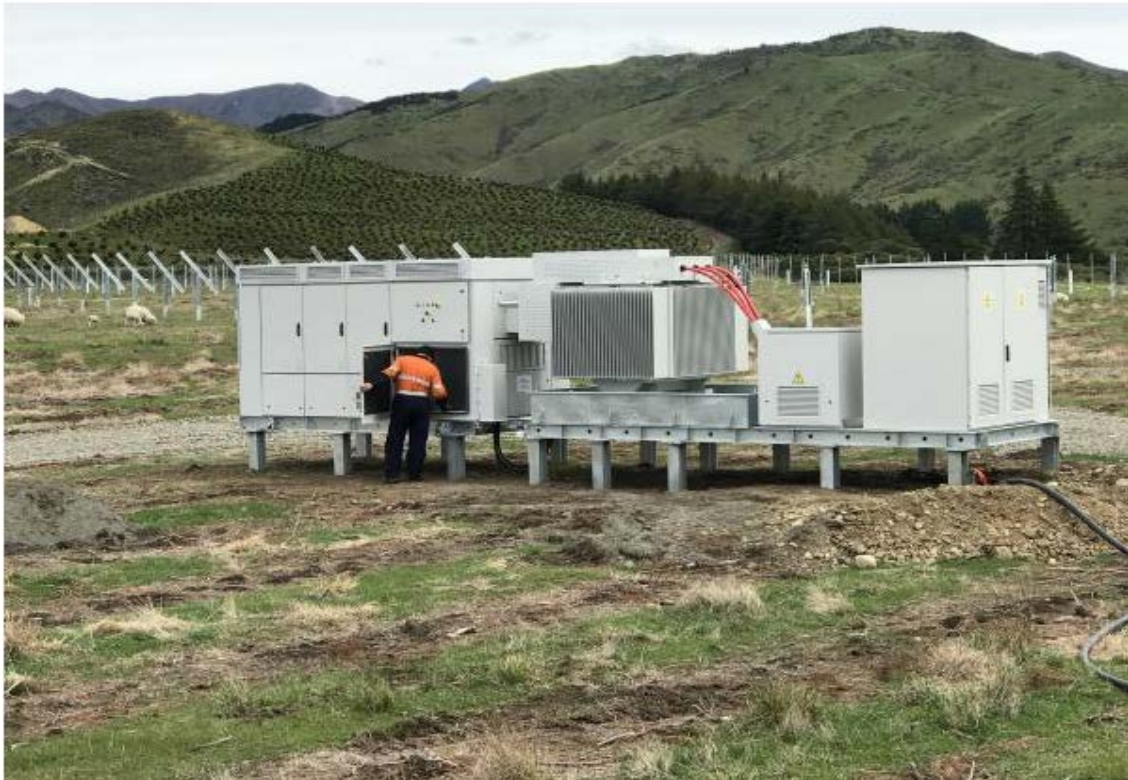
Figure 3: Photograph of HEMK MV skid gen 3 (source: Infratec).
