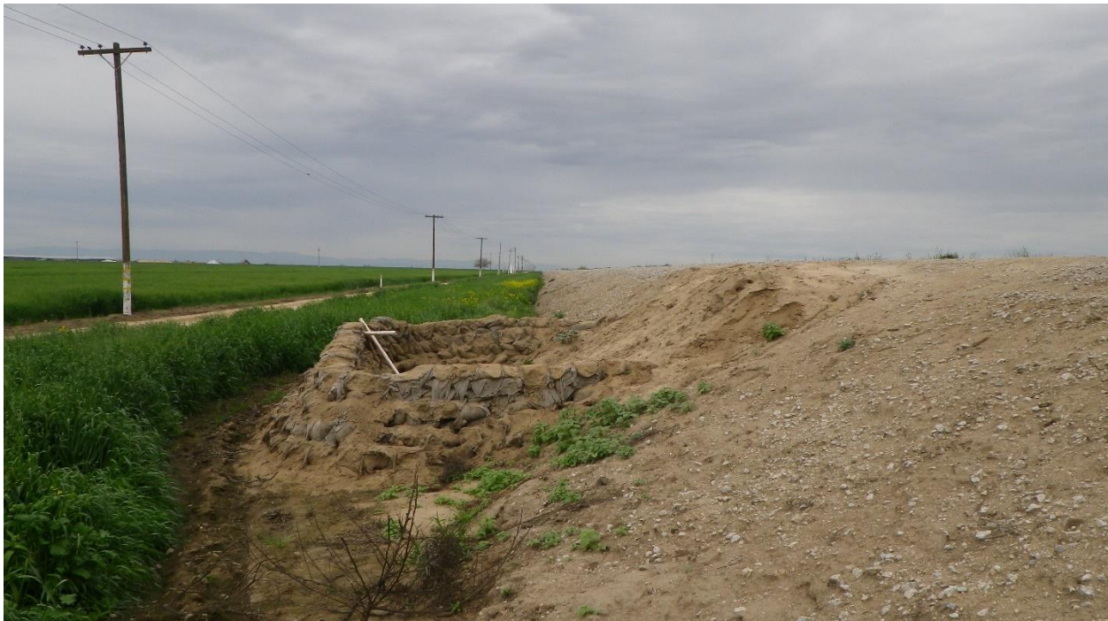
Figure 4-47 2011 Fresno River Levee Boils
