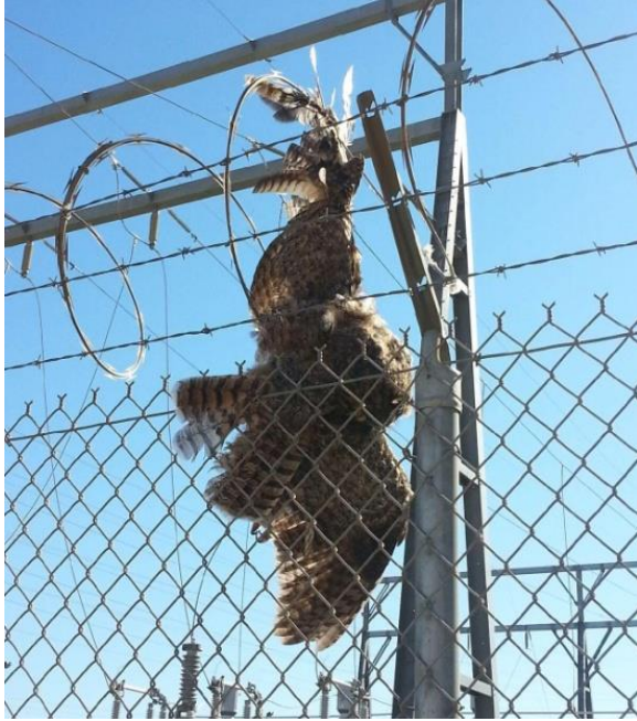
Photo 8. A great-horned owl died after becoming entangled on the razor wire placed on top of this cyclone fence surrounding a substation in Alameda County. Photo by Joanne Mount.
