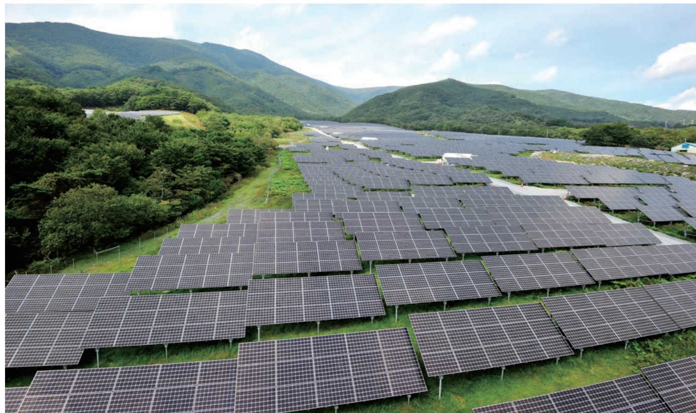
Goyozan Solar Power Plant (Ofunato-shi, Iwate)
