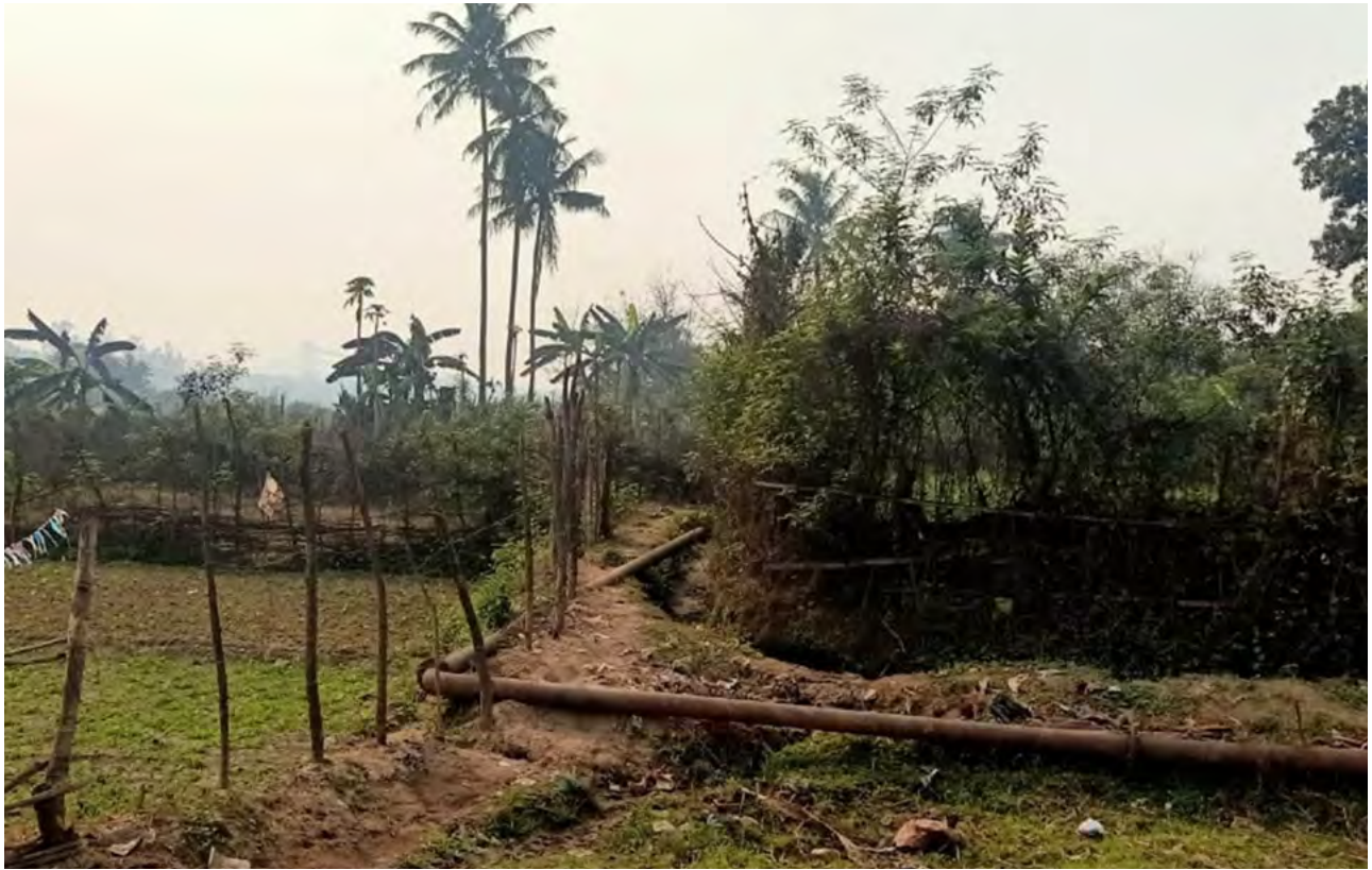
Water Pipeline for community supply at Talcher Area
