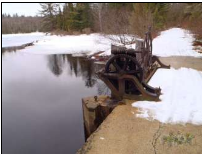
Flow control gate at the Seboeis Lake Outlet Dam.
