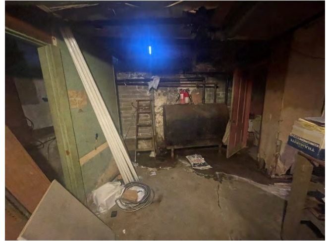
Description: Pawn Shop Basement, Sample AS-2 location
