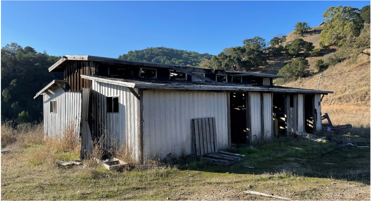
Photo 5. Exterior view of the dilapidated barn in the Study Area, south of the California bay woodland community. Facing northeast; photo taken on November 28, 2023.
