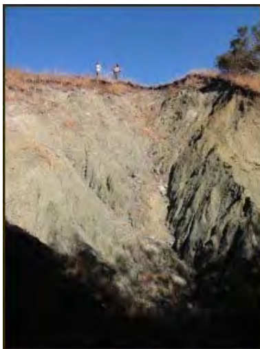
Before photo of biotechnical repair in Olema in Point Reyes National Seashore.
