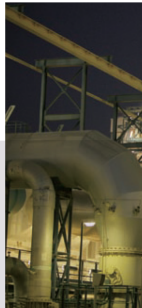
The TAWEELAH B power station in the U.A.E. began commercial operations in October 2008
