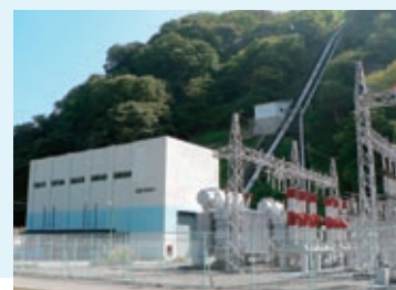
Mibugawa Power Plant
