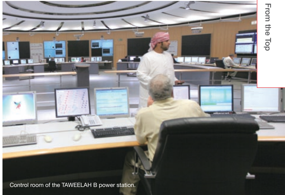
The Taweelah B power station in the U.A.E. (pictured at night) began commercial operations in October 2008
