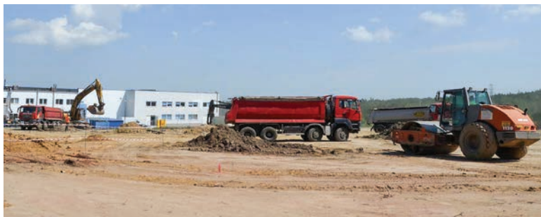
Tristone closed its North Carolina facility just two years after opening it. Here, construction crews work on the building in 2018.
