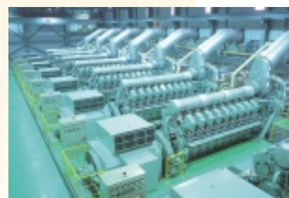
Diesel Power Plant of the Taiheiyō Energy Center
