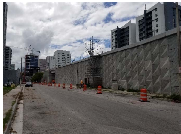
6. NE 11 th Street, south side shows above grade construction of rail line heading toward Government Center.
