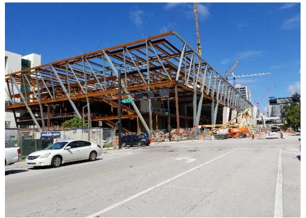
5. Overtown Metrorail station undergoing redevelopment for Miami Central Building and Brightline / Tri-Rail station.
