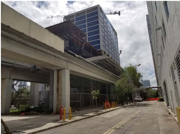
9. Existing Overtown Metrorail station with incoming Miami Central Building construction on top.
