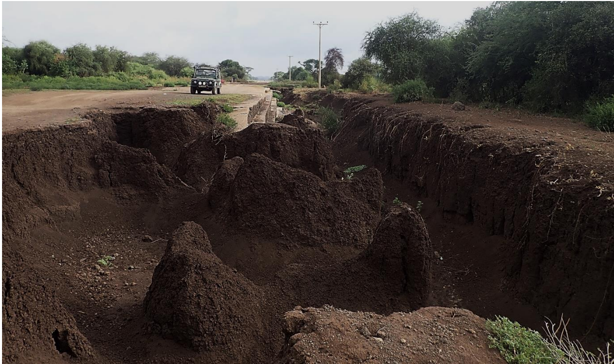
Figure 1-2 Poor stormwater management of the existing Illasit-Taveta Road resulting in severe erosion and gully formation with the Rombo section of the road.
