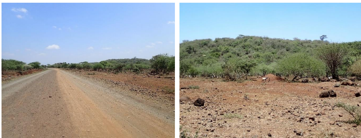
Figure 4-5 Illasit-Taveta road where it passes through relatively natural habitat comprising Acacia-Commiphora deciduous bushland and thicket (left) with some impacts experienced from livestock (right)
