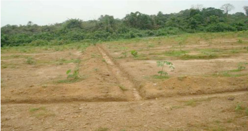
Figure 3: various runoff ditches put in place by BR Fuel but which has been structured differently by continuous and heavy water flow.
