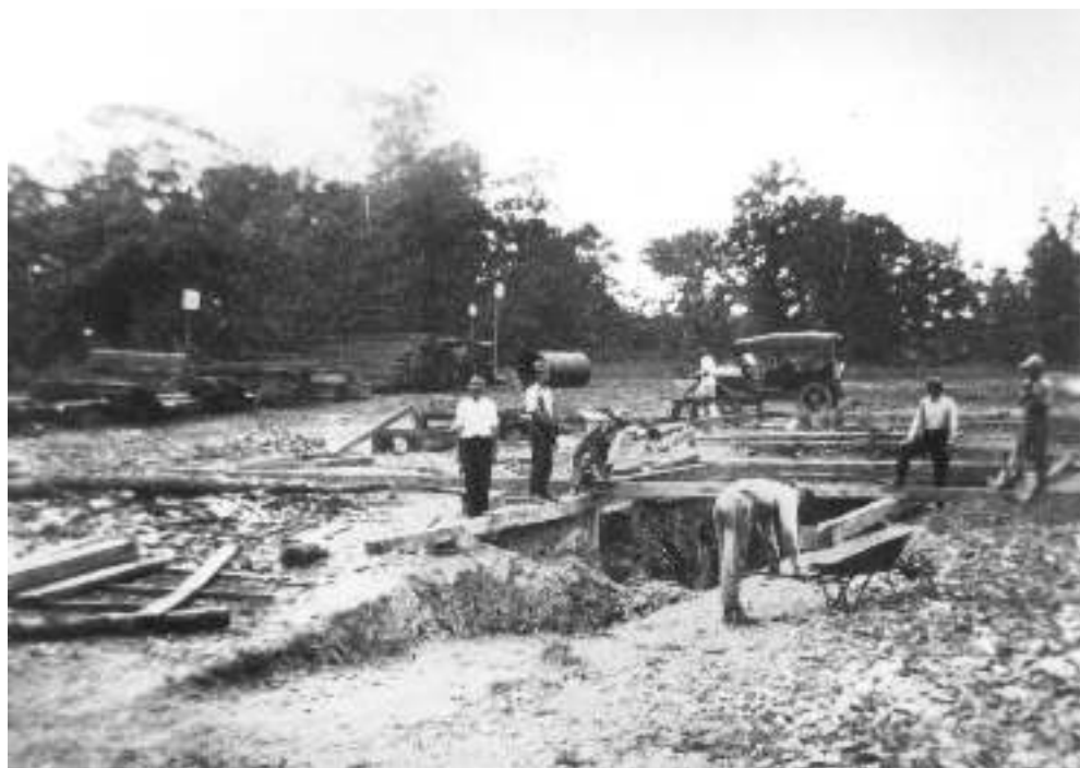
Overview of the Choate Mine entrance area as renovation commenced in the summer of 1917.
