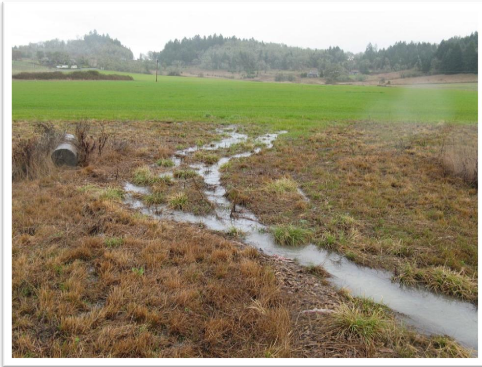
Figure 3.6. (After) Water from adjacent property that previously flowed NW down 'Cantrell ditch' (out of photo to left) is now diverted down swale 5 to the center of the East Phase. February 2012
