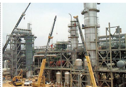
METOR is currently constructing an 850,000 ton/year facility adjoining an existing plant that is capable of producing 750,000 tons of methanol a year. Commercial operations at the new facility are scheduled to begin in the first quarter of 2010.
