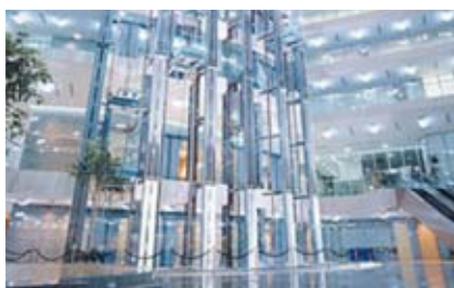
Elevators at the headquarters building of the Securities Commission of Malaysia. MC helped supply 12 elevators, including observation elevators, with glass walls for this building.
