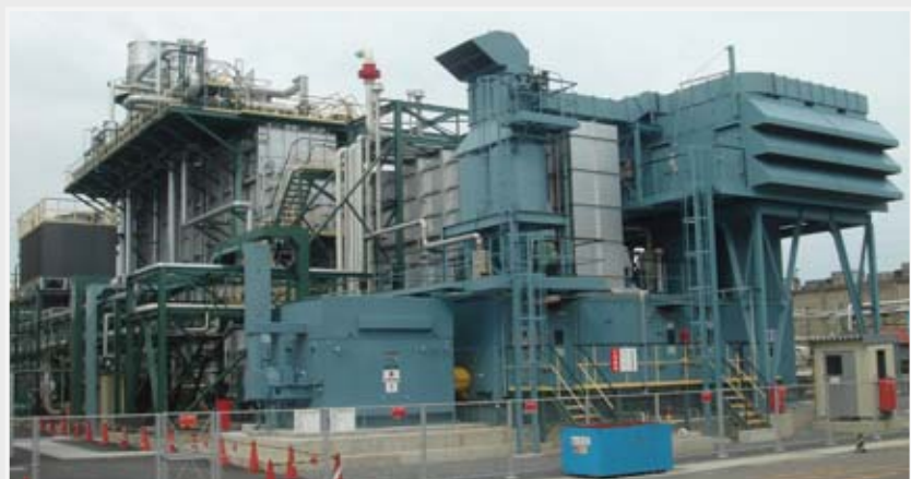
This natural gas-fired cogeneration facility was installed at JSR's Yokkaichi Plant (Construction completed in April 2010)
