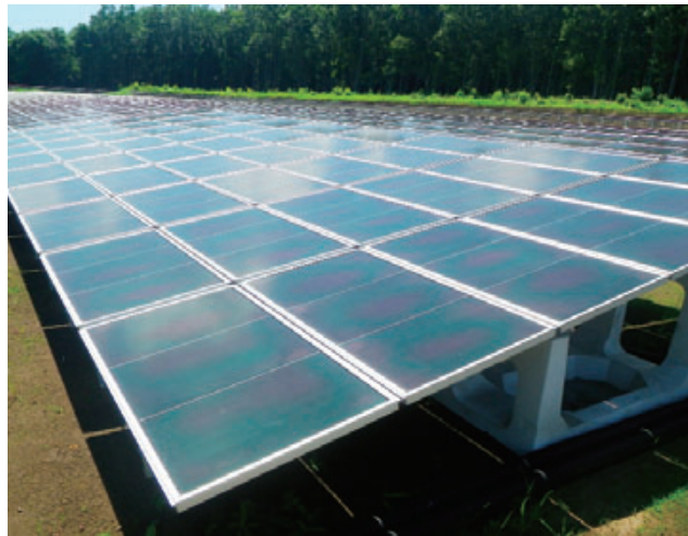
This photovoltaic power plant in Kumamoto is the first mega solar project MC has built and is operating in Japan.
