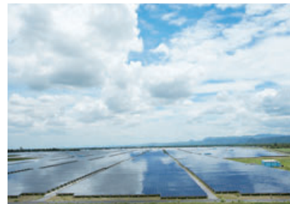
This solar photovoltaic project in Lop Buri, Thailand, started operations in May 2013. It produces approximately 84 MW of electricity, making it one of the largest such projects in the world. MC has an approximate 33% equity interest in this project.
