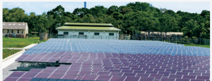
A solar photovoltaic power generation system, currently the largest in Southeast Asia (Brunei).
