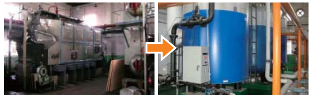
Before conversion: Coal boiler After conversion: Natural gas boiler
