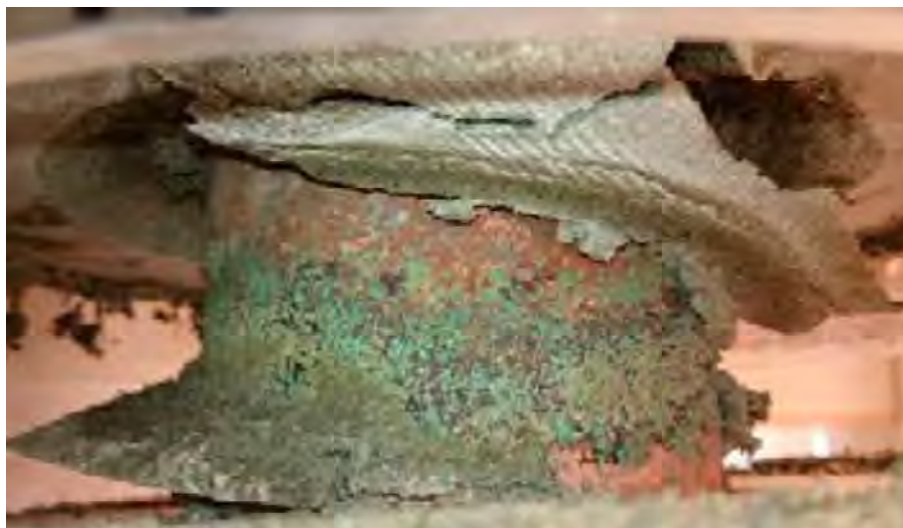
Figure 2.8. Detail from Figure 2-27 in TR 15-09. Severe corrosion of the copper heating tube after only seven days of laboratory exposure that at least reminds of the true Sauna effect, i.e. with only indirect contact with 0.6M chloride solution.
