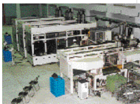
Household appliance recycling plant
