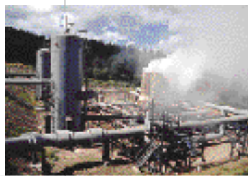
Sumikawa geothermal plant
