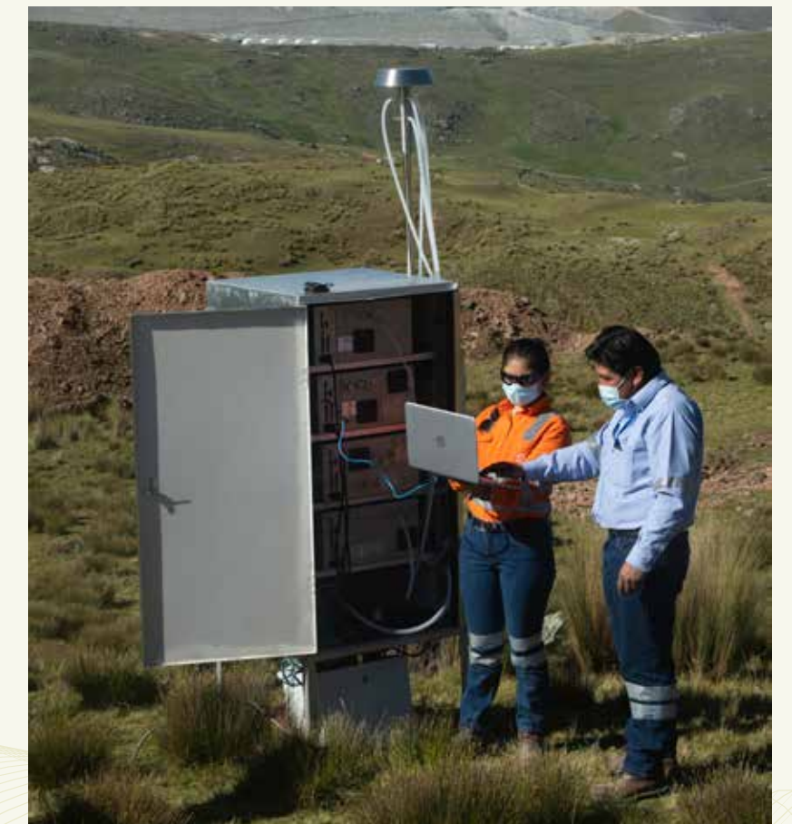
Environmental monitoring station
