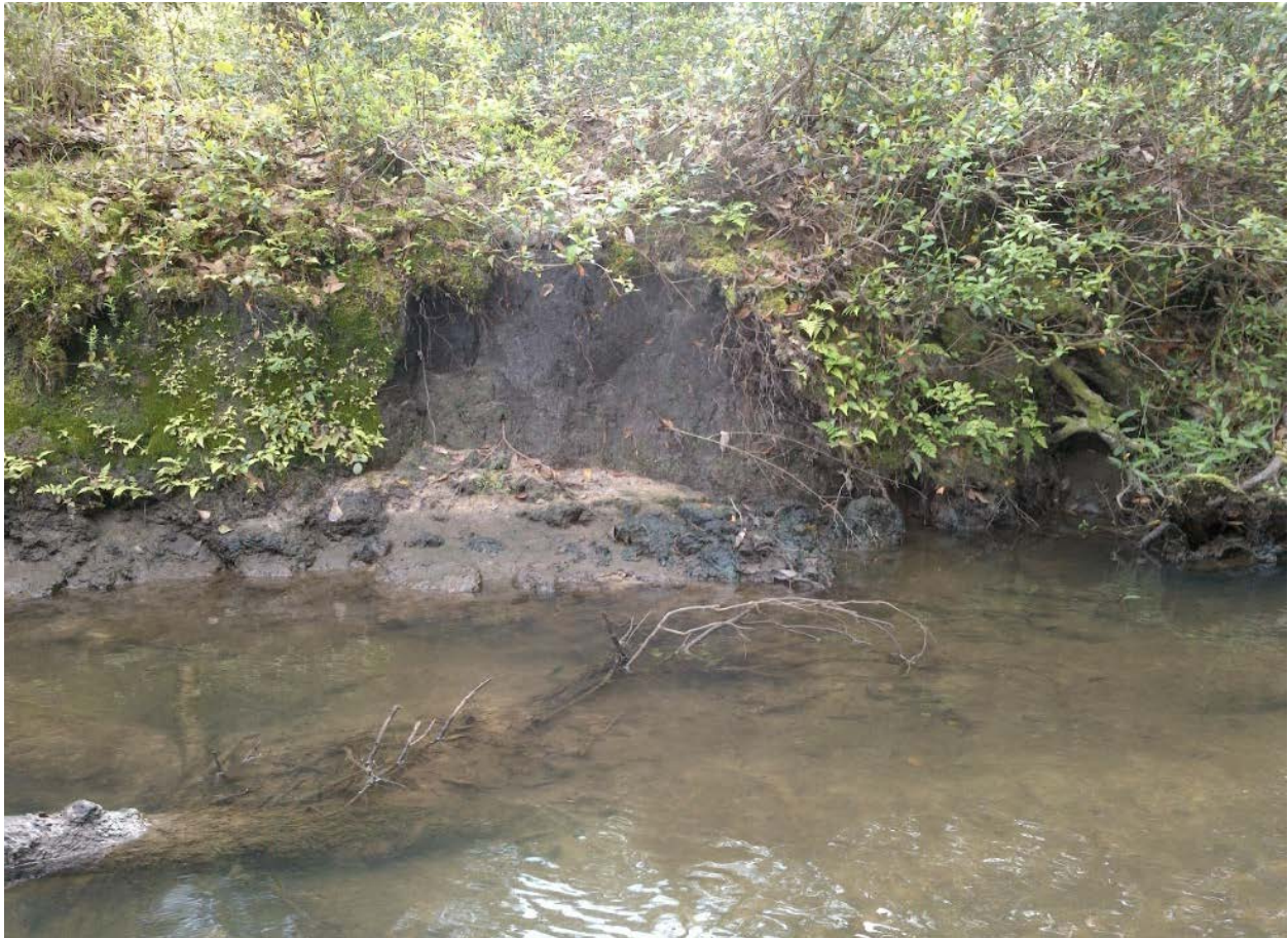
Figure 7.8 Bank Sloughing Along Wolf Creek
