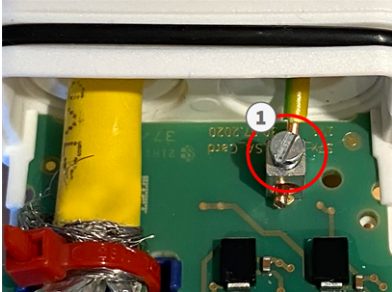
Fig. 19: Ground wire connected to terminal
