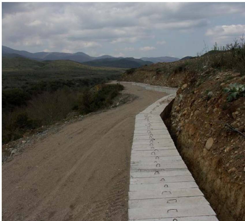
Photo 69. Newly constructed irrigation system which intersects with the route of highway alignment 2 (near village Miravci).
