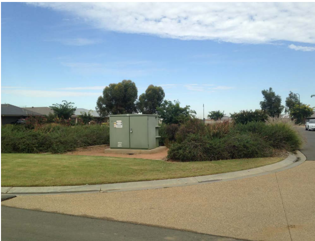
Screen planting and gravel access area around substation
