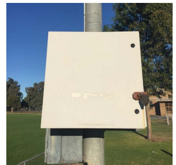
Irrigation cabinet example
