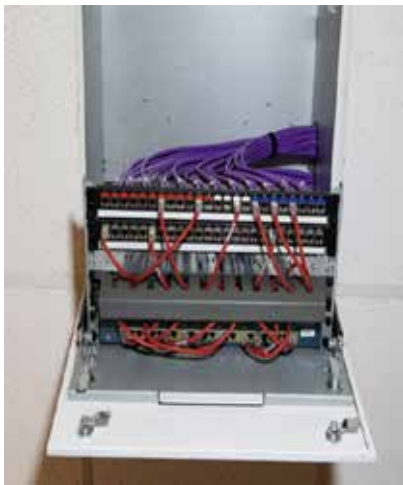
Active equipment installation
