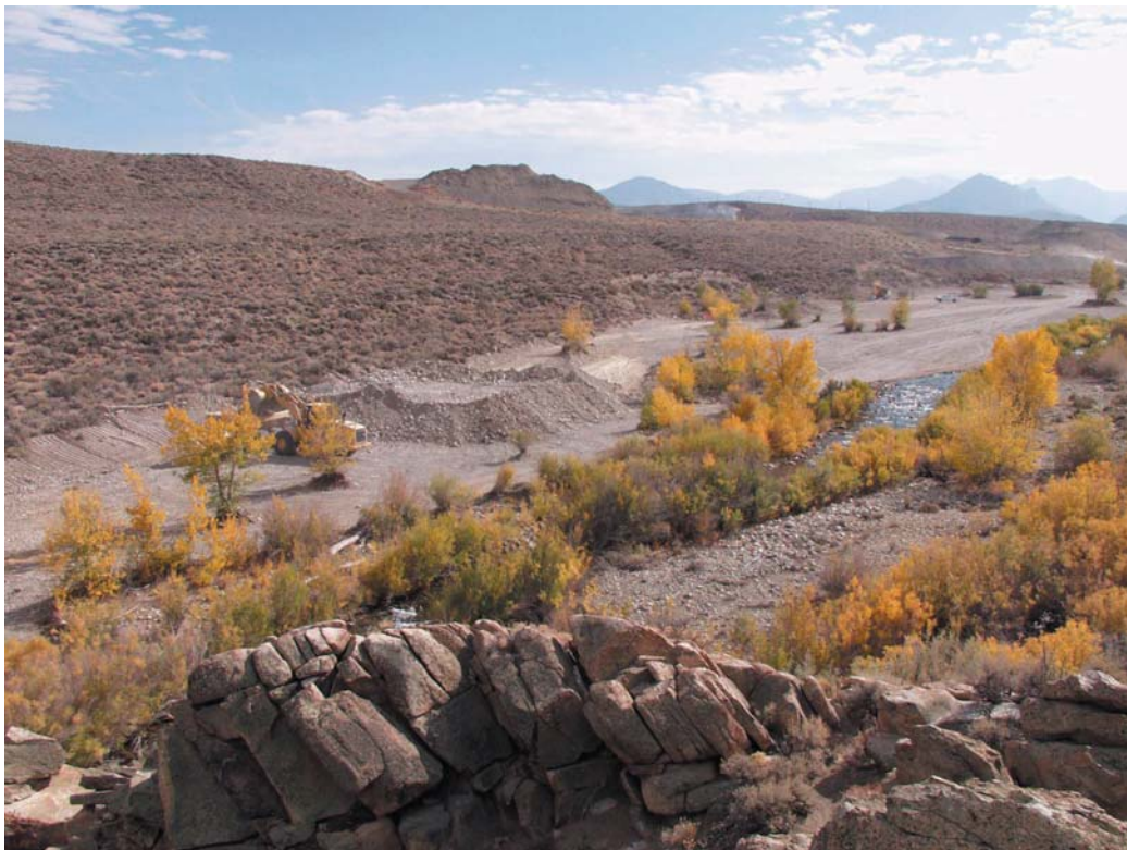
Figure 7. Photograph of the 3D Floodplain Restoration site, taken from the Narrows after the floodplain excavation was nearly completed.
